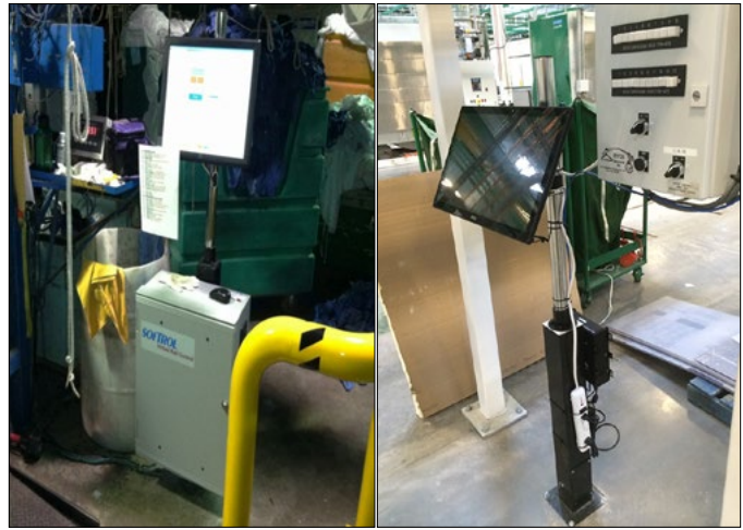
Figure 2. Left: A typical lift station. Right: A typical call-off station.
